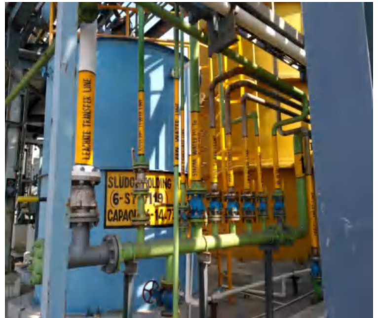
Close loop effluent transfer system for effluent collection
