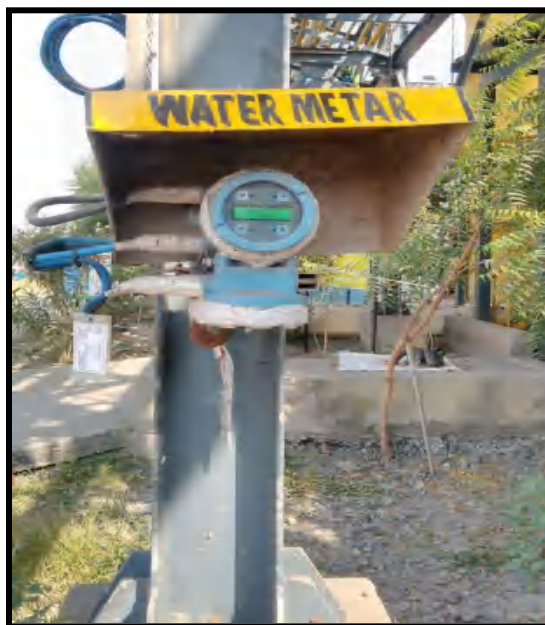
Flow Meter at RO Inlet (CT Blowdown)
