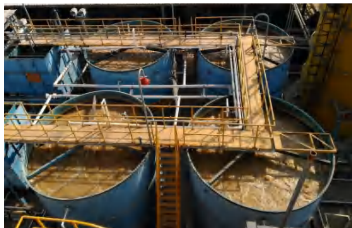
Effluent Treatment Plant capacity: 125 KLD
