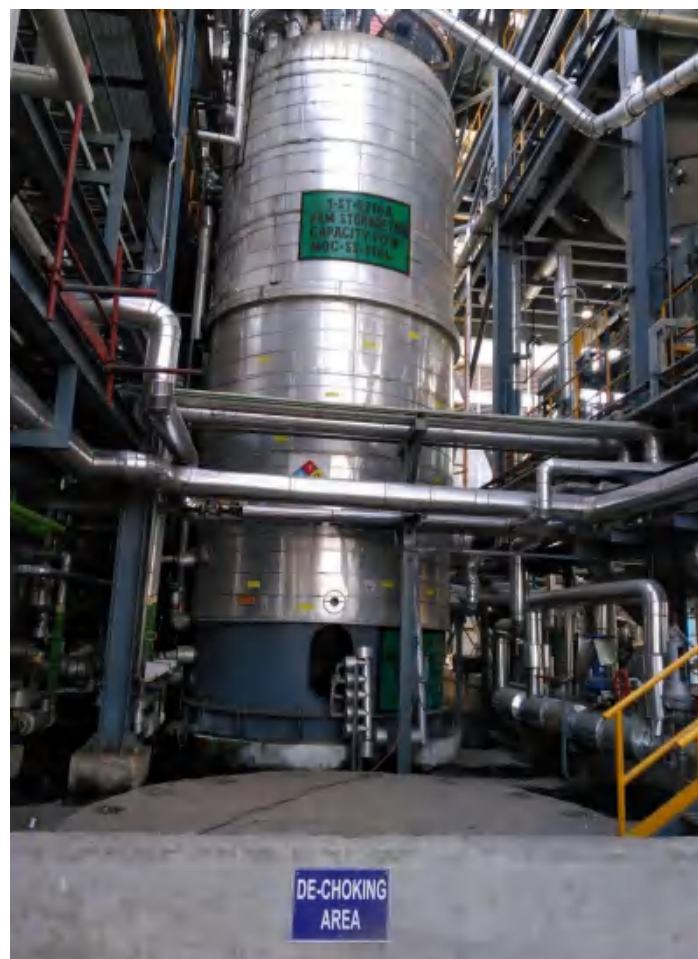
Photo of raw material storage area with required de-choking facility
