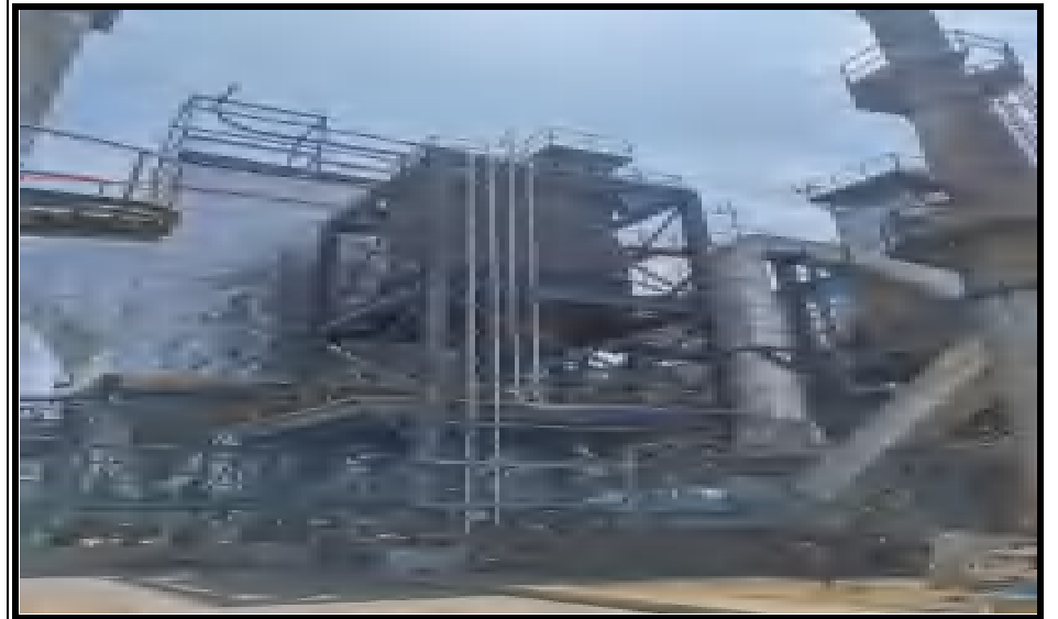
Silo installed for fly ash storage and dusting free truck loading
