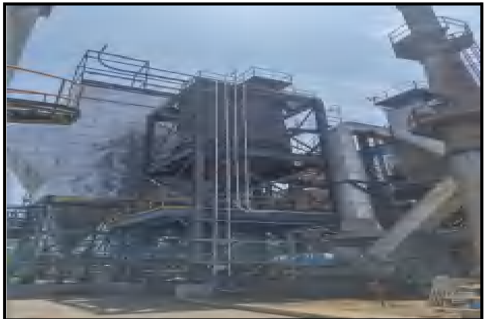
Silo installed for fly ash storage and dusting free truck loading
