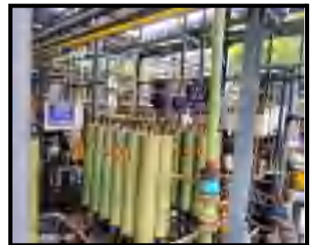
Utility RO-1 - 150 KLD & Utility RO-2 - 550KLD
