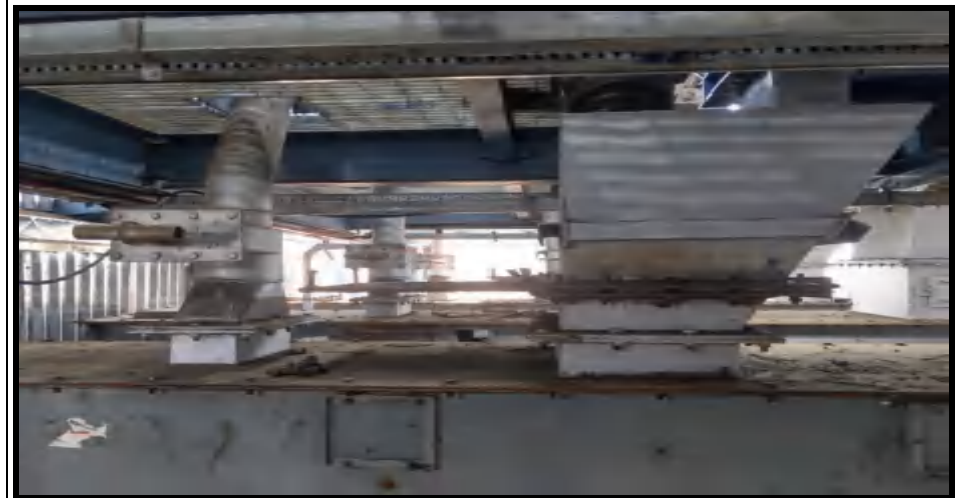
Automated Lime feeding system for controlling SOx commission.
