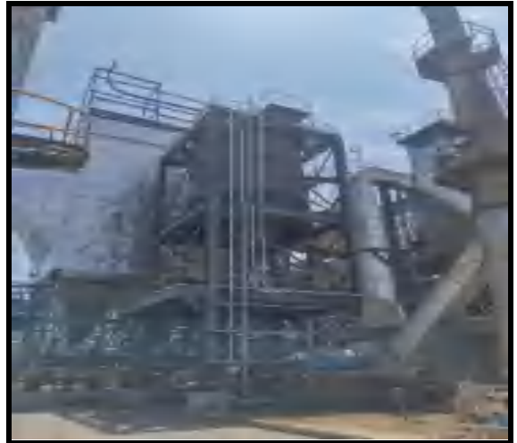
Silo installed for fly ash storage and dusting free truck loading
