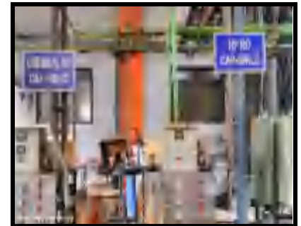
RO Process (Chemical)-60 KLD & HP RO-50KLD
