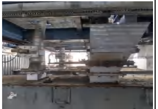
Automated Lime feeding system for controlling SOx commission.
