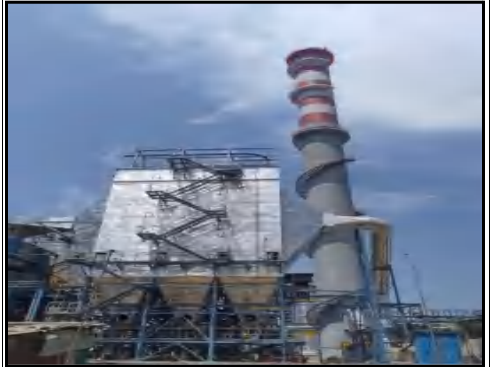
3 stage ESP and 76 m stack attached to boiler
