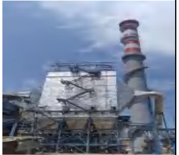
3 stage ESP and 76 m stack attached to boiler
