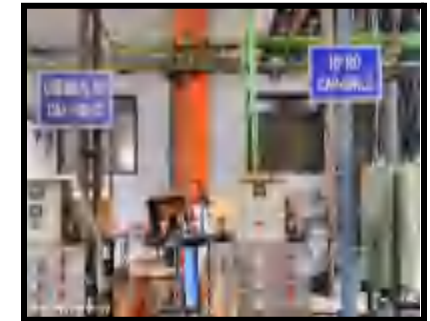
RO Process (Chemical)-60 KLD & HP RO-50KLD
