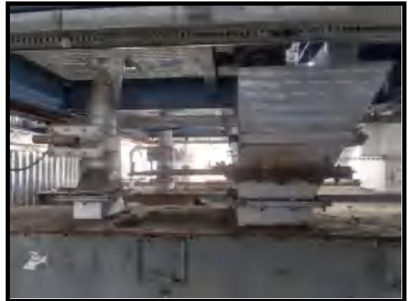
Automated Lime feeding system for controlling SOx commission.
