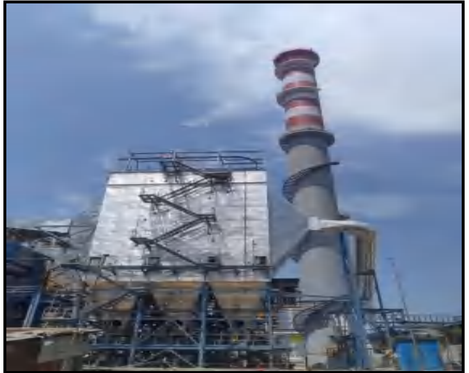
3 stage ESP and 76 m stack attached to boiler
