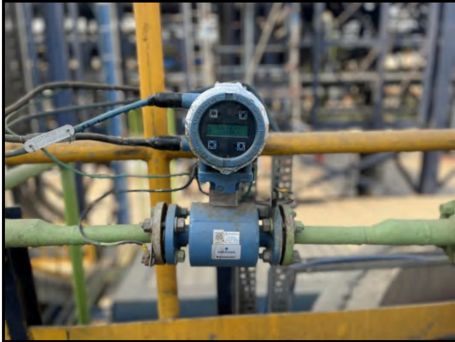
Inlet of ETP
