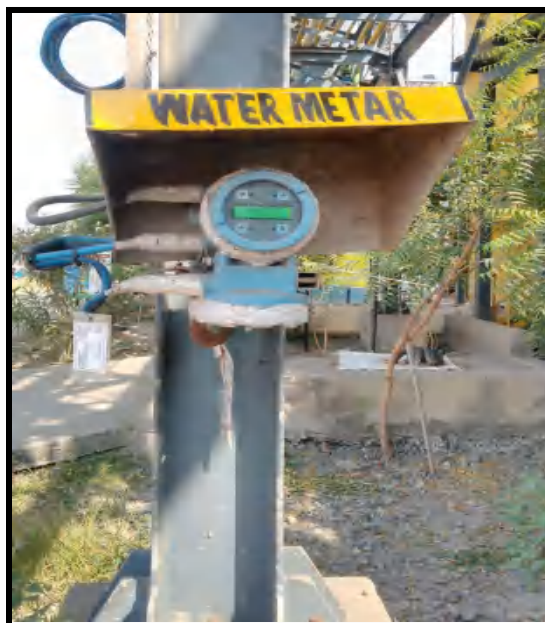
Flow Meter at RO Inlet (CT Blowdown)
