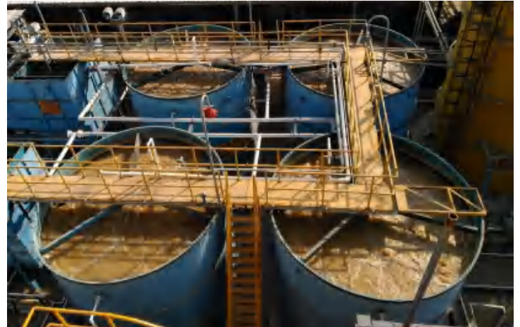
Effluent Treatment Plant capacity: 125 KLD
