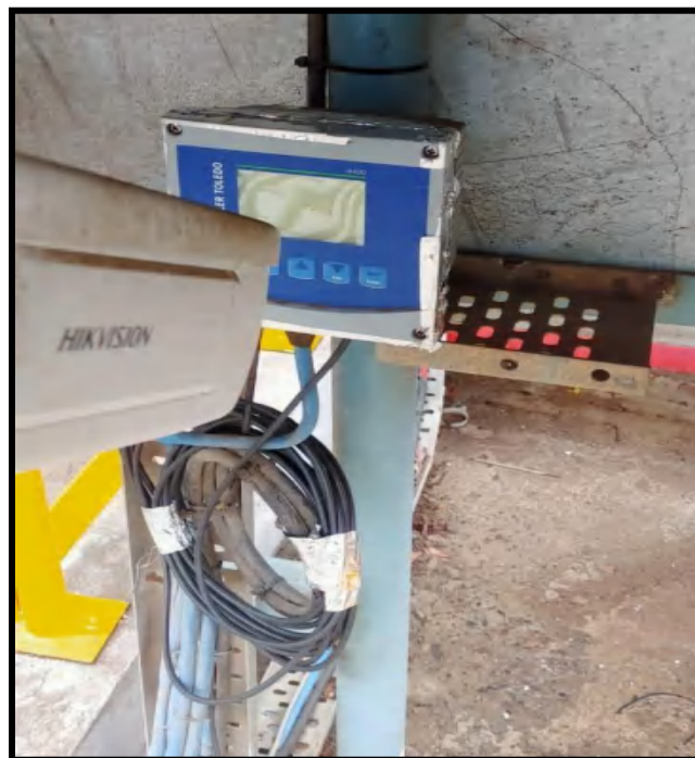
Flow Meter at the ETP Outlet (GIDC Discharge)
