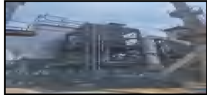
3 stage ESP and 80 m stack attached to boiler
