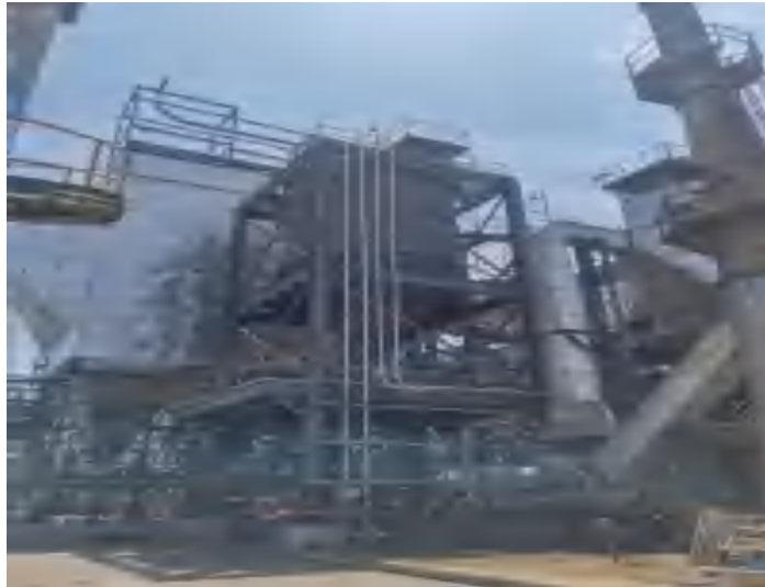
Silo installed for fly ash storage & dusting free truck loading
