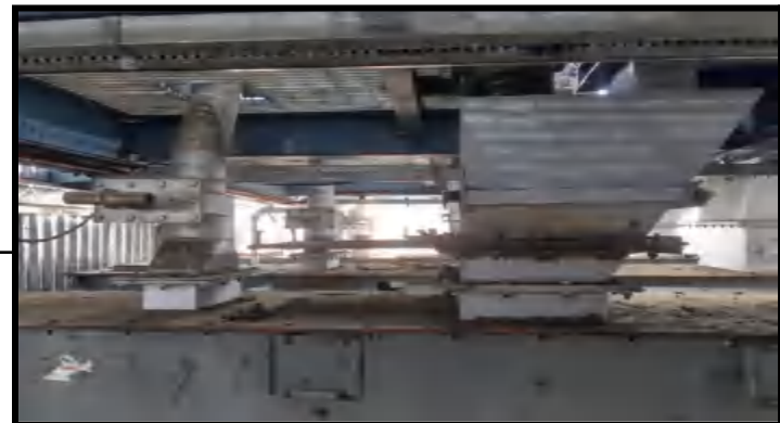
Silo installed for fly ash storage & dusting free truck loading
